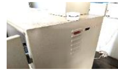
UPS temp. monitor
